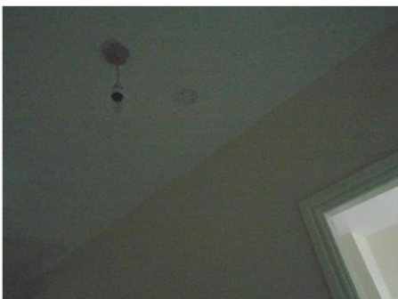
Missing smoke detector
