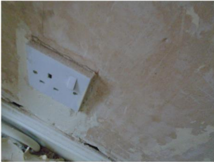
Socket identified in bathroom
