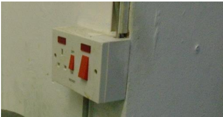
Cooker switch installed
